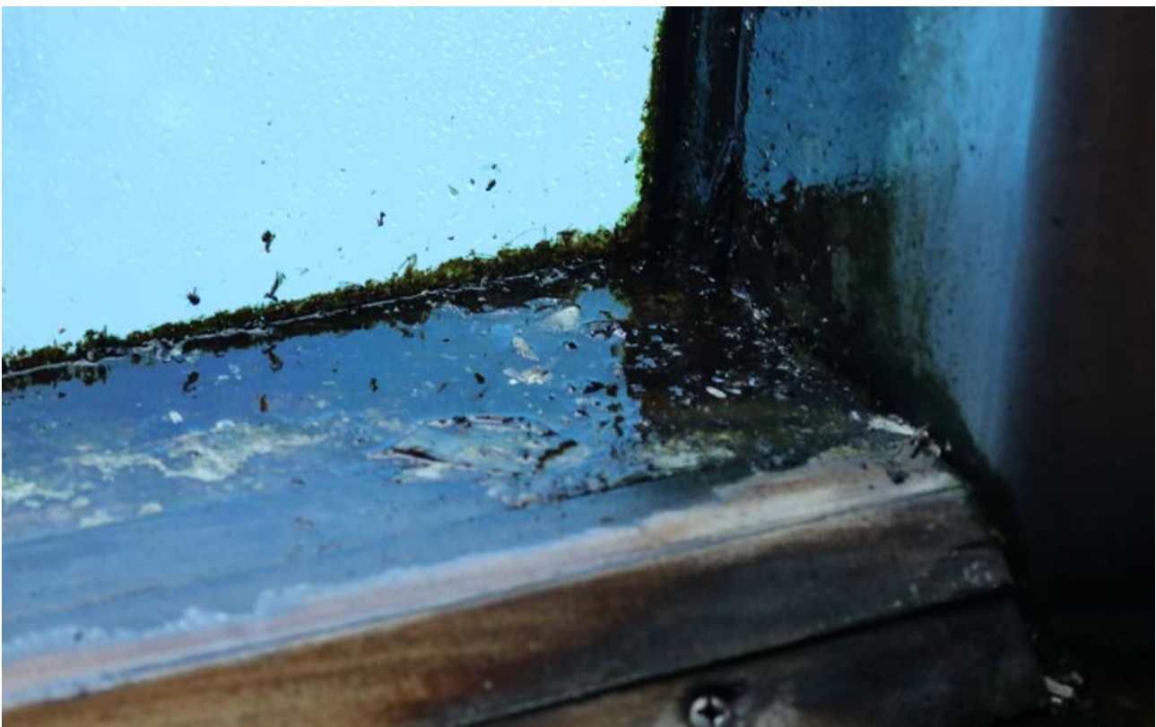
Figure 44. One of the many leaks in the underwater viewing areas at MarineLand, note the build-up of algae and other detritus. This area clearly hasn't been cleaned for a significant amount of time. Photo supplied by One Voice (taken 8 October 2021).
